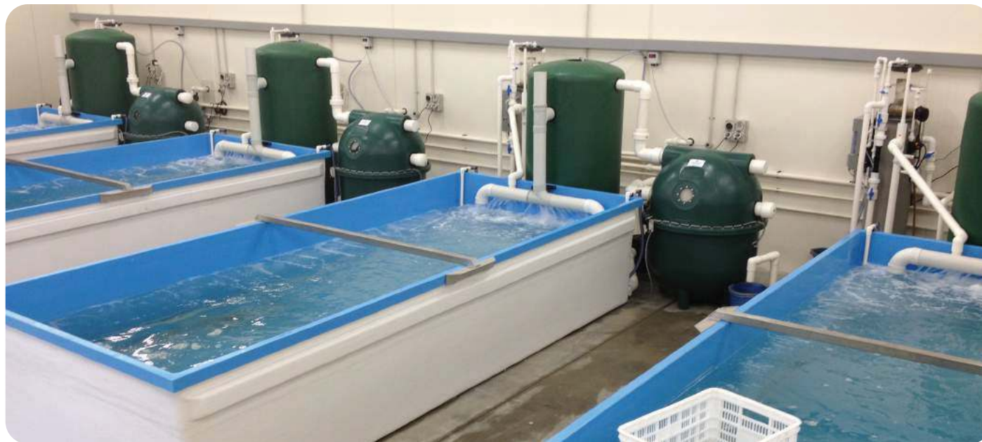
PG filters in an aquaculture facility
